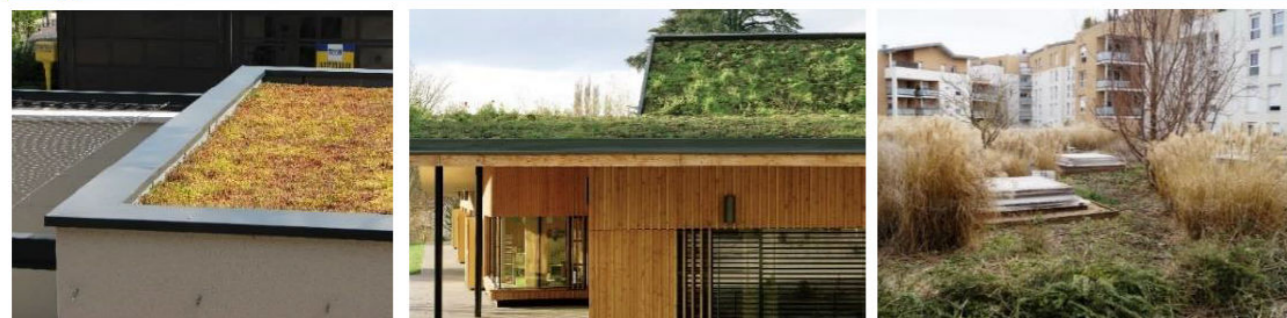
Toiture extensive (substrat 6cm) Toiture intensive (substrat 12 cm) Toiture intensive (substrat 50 cm) Source : Ademe
